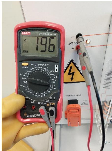
Service plug installed
